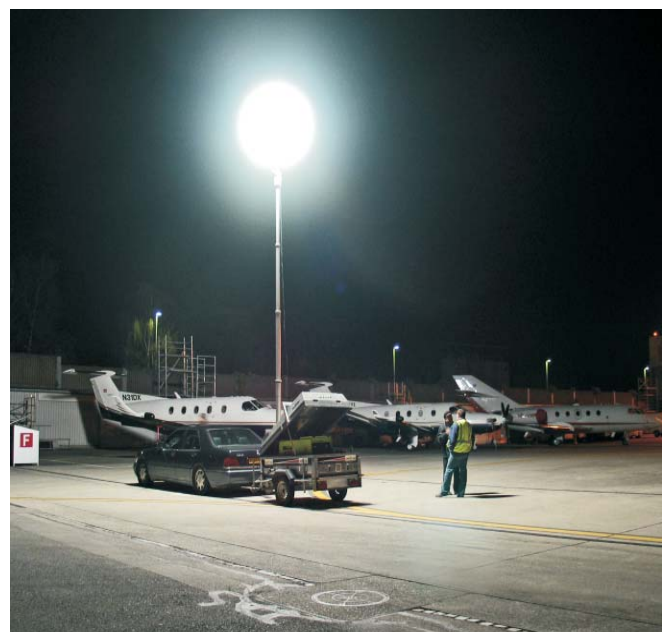
Lumitrail 4000 - Baustelle aeroport
